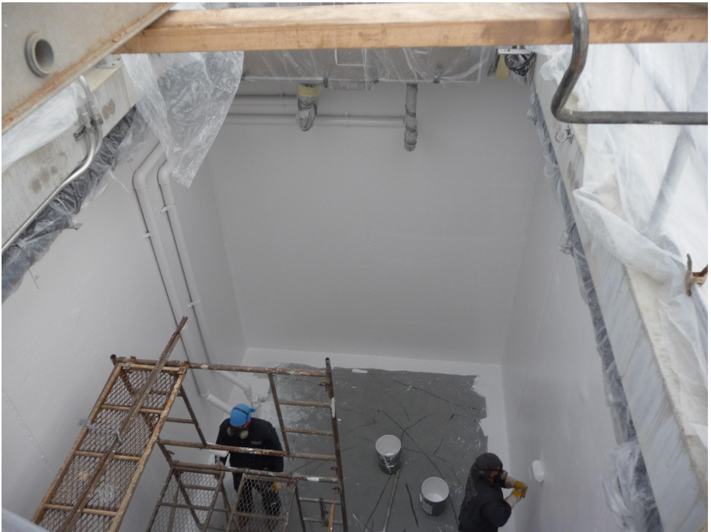
Subcontractor IK Stoltzfus Applying Primer to the Equalization Tank at the Frystown WWTP
