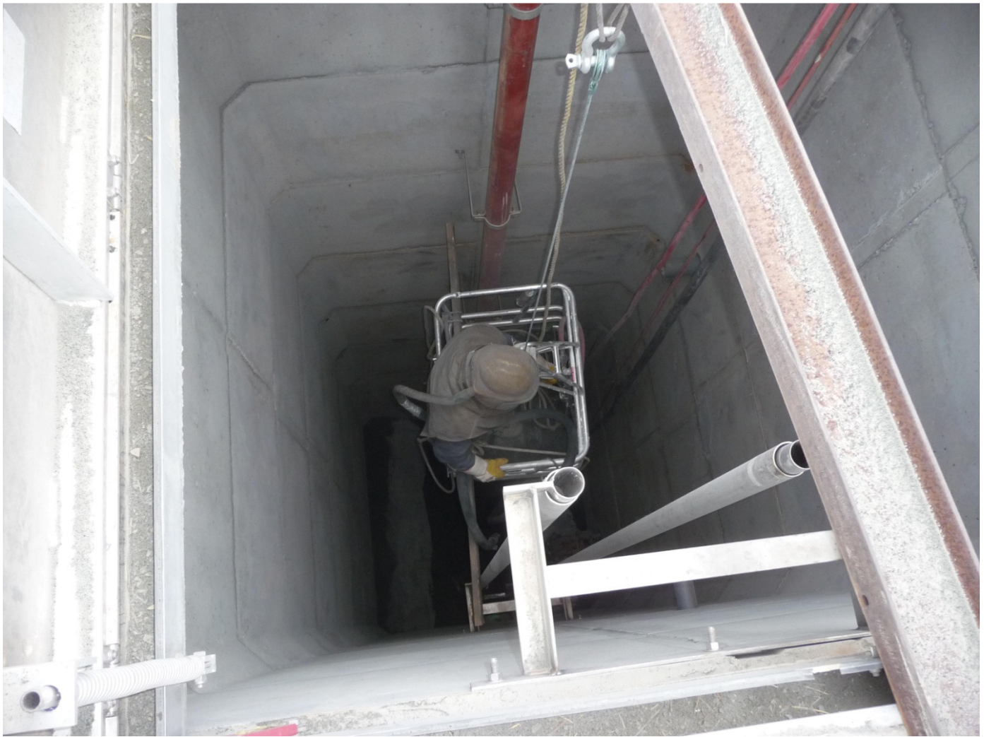
Subcontractor IK Stoltzfus Sandblasting the Concrete Surface of the Wet Well at Fzystown WWTP
